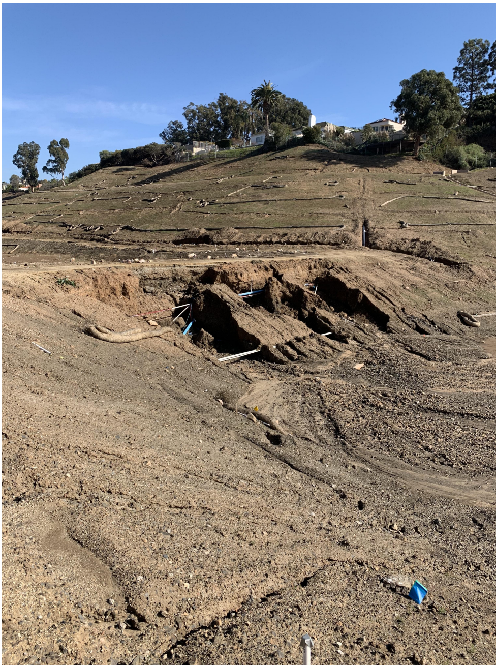
Photo 1: Looking northeast at the Basin 9 berm after the December storms. Severe erosion caused collapse of the berm and washed mud into the basin.
