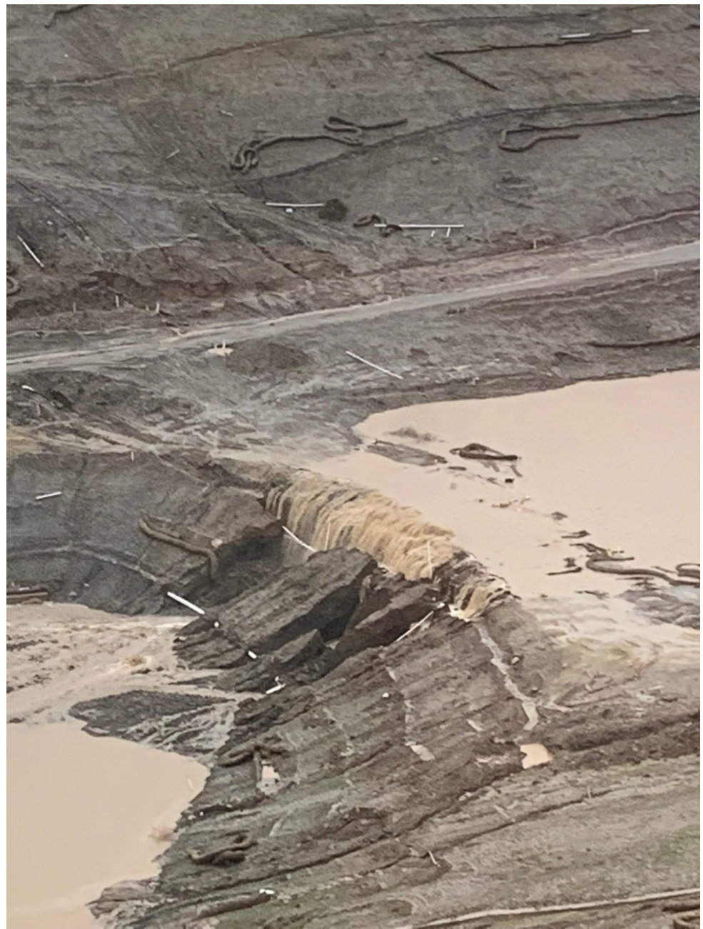
Photo 2: Looking west at the berm between Basin 8 and Basin 9, taken during the December storms. A period of intense rainfall resulted in a washout on the slope of the berm.
