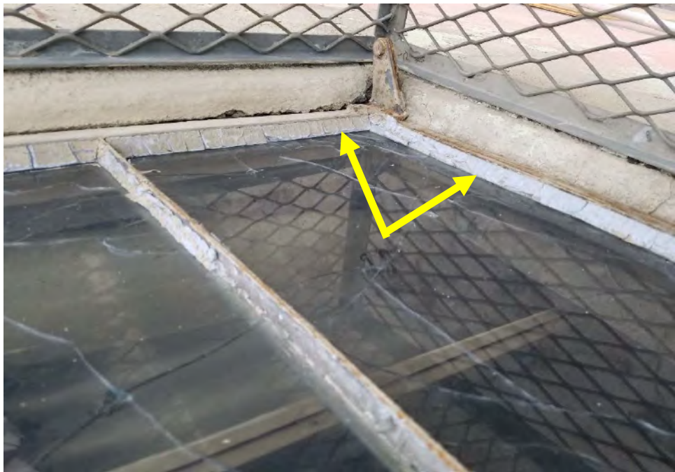
Photograph 2: Building 1: view of asbestos-containing window putty.
