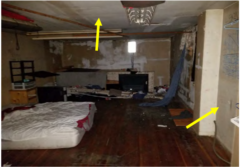
Photograph 7: Building 1: view of asbestos-containing button board (plaster/drywall) throughout walls and ceilings.
