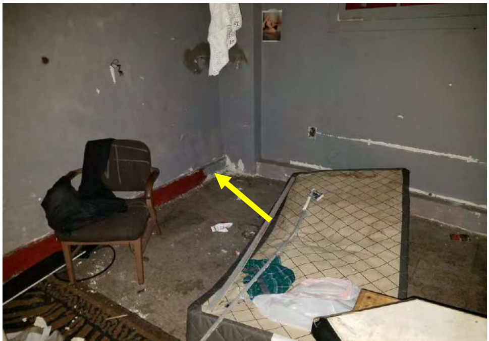
Photograph 4: Building 1: view of asbestos-containing baseboard plaster.
