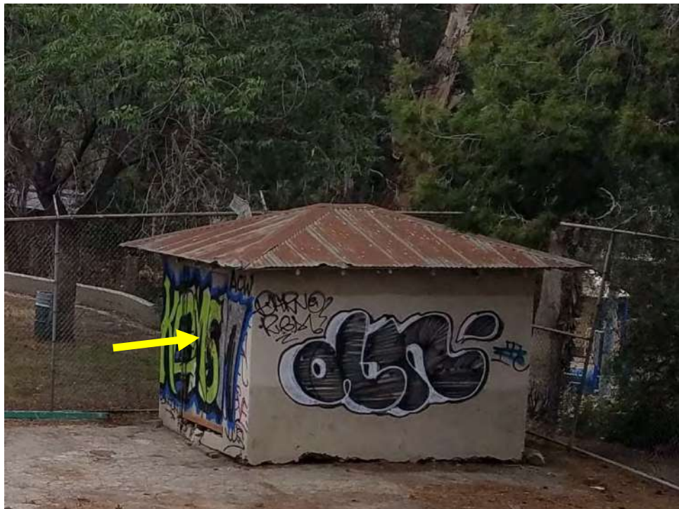
Photograph 14: Shed 1: view of lead-containing main door.
