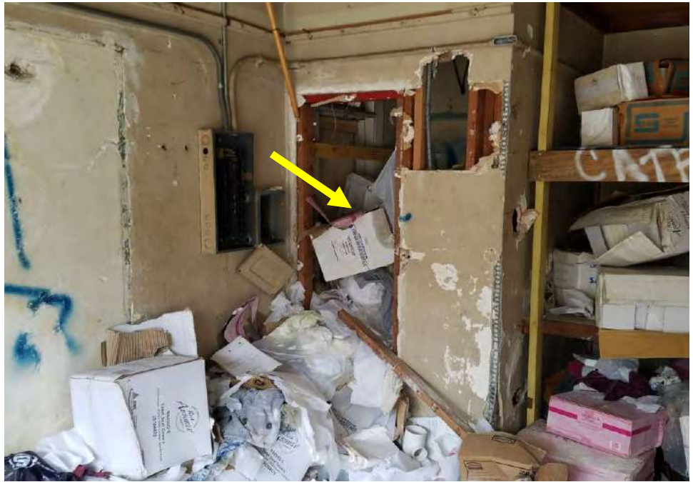
Photograph 12: Building 2: view of restroom with lead containing sink and toilet.
