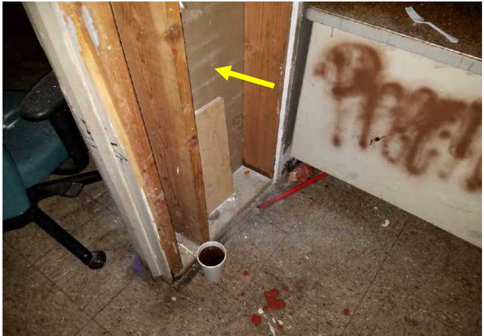
Photograph 8: Building 1: view of asbestos-containing joint compound associated with drywall.
