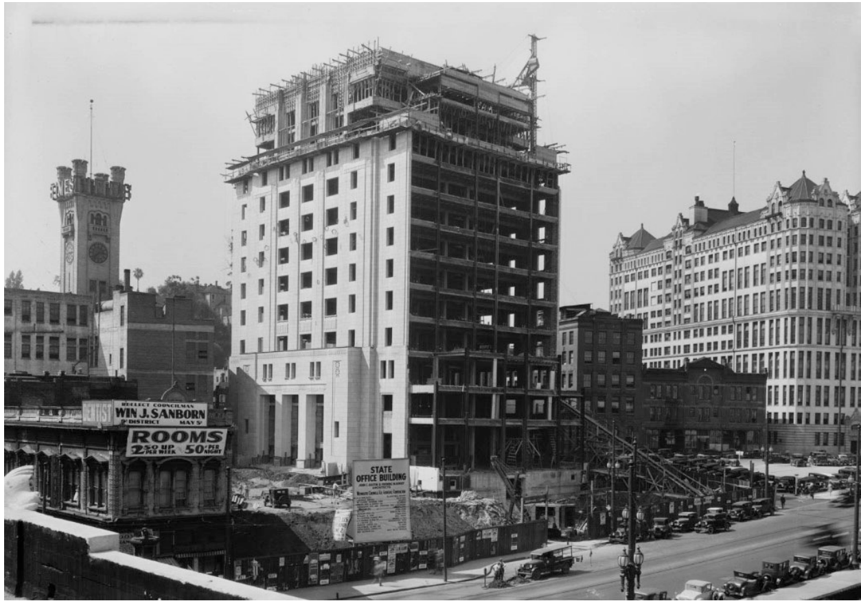
Plate 2. California State Building under Construction; Larronde Block (left) and second Times Building (left, background), 1931. View northwest from intersection of Spring Street and 1st Street (Water and Power n.d.).
