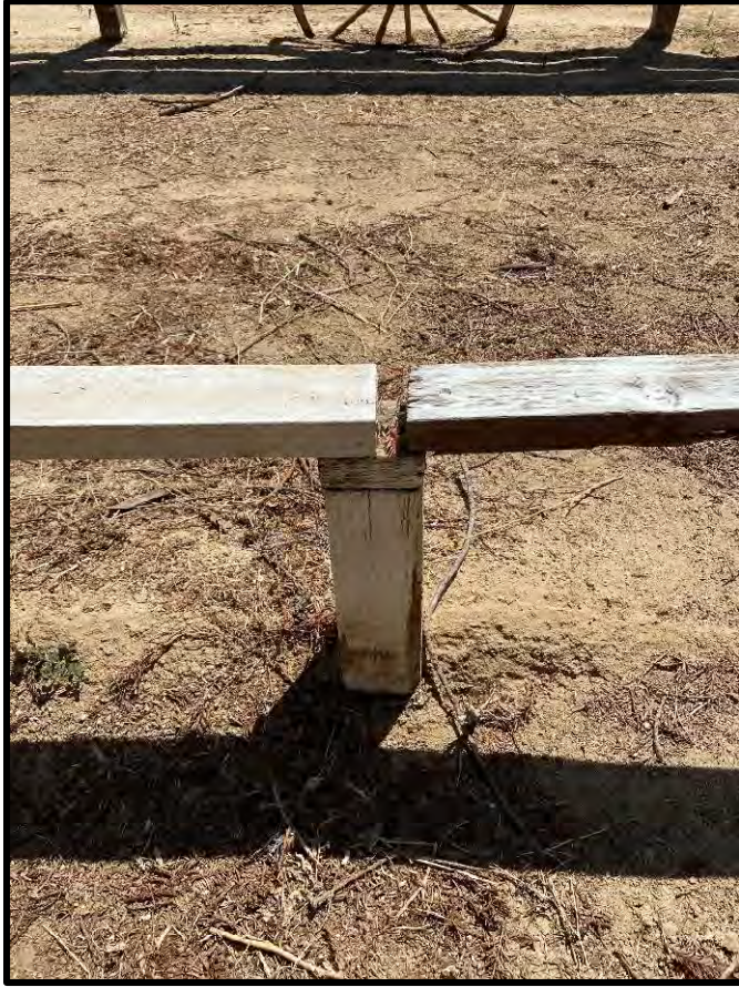
Figure 42 Deteriorated connection at the Internal Guide Rails.
