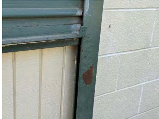
Detail of paint loss and corrosion at metal frame (ARG, 2023).
