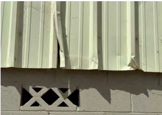
Typical damage at base of metal cladding (ARG, 2023).
