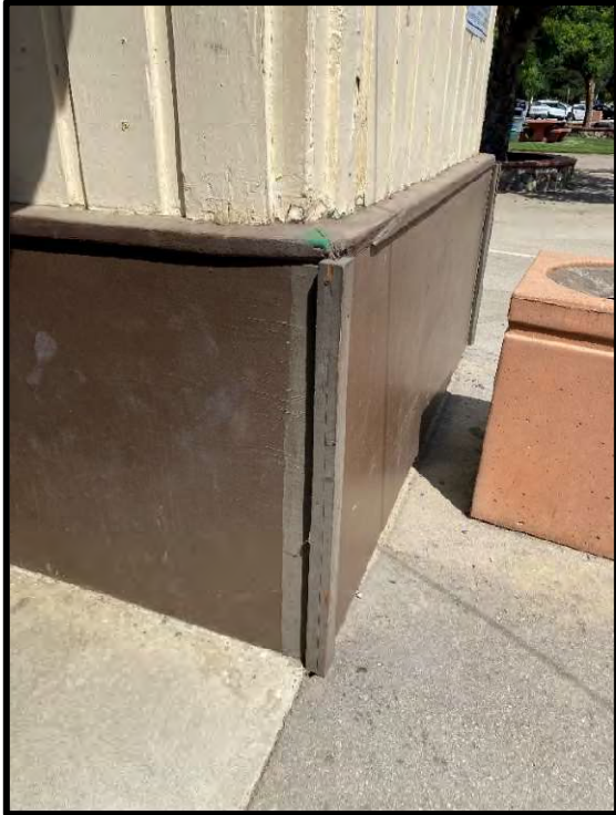
Figure 19 Close up of the Ticket Booth top vertical siding and bottom wood panels.
