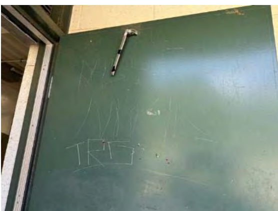
Detail of scratches at restroom door (ARG, 2023).
