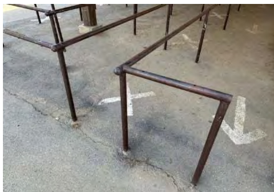
Stanchions and directional markings at asphalt pavement; note cracks and missing end cap (ARG, 2023).
