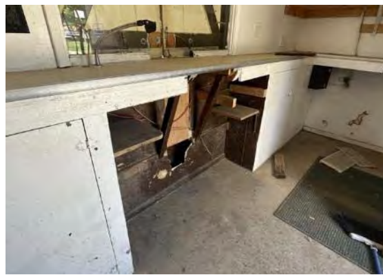
Detail of wall damage below ticket window (ARG, 2023).
