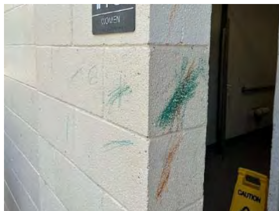
Detail of graffiti at CMU wall (ARG, 2023).
