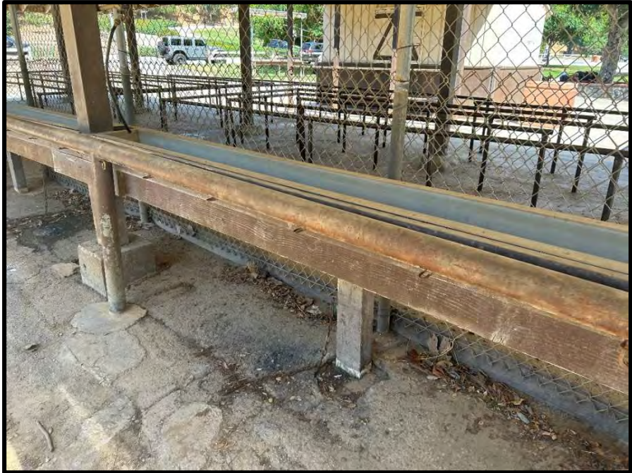
Figure 17 View of the steel framing at the south side of the canopy.
