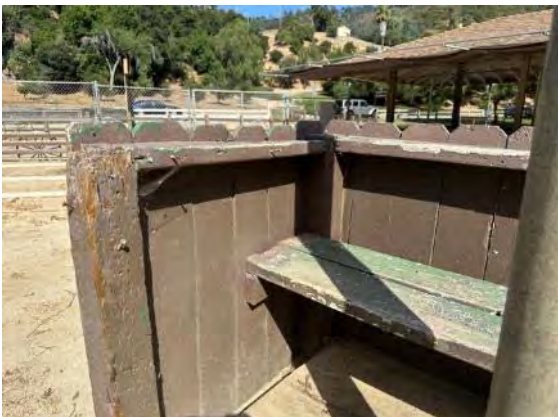
Detail of employee stand; note chewed wood post and weathered paint finishes (ARG, 2023).
