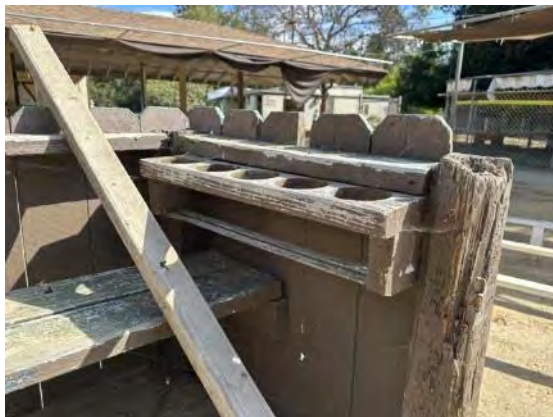
Detail of cup holders at stand; note termite damage at wood post (ARG, 2023).
