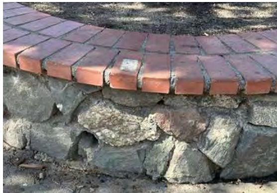
View of planter wall; note gaps in stone masonry and eroded joints (ARG, 2023).
