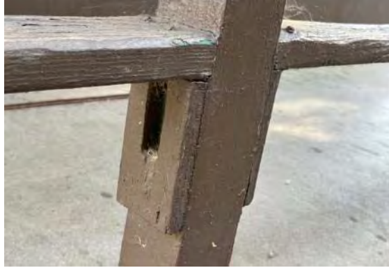
Detail at porch top rail; note wood bracket from previous railing (ARG, 2023).
