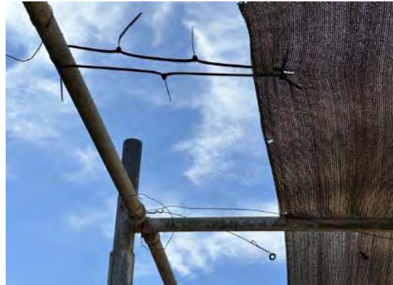
Detail at canvas awning; note tears and zip ties (ARG, 2023).
