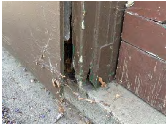
Detail at door frame; note heavy wood decay/loss at frame and wall (ARG, 2023).
