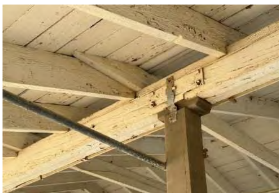
Detail at column; note metal strap repair at connection plate (ARG, 2023).
