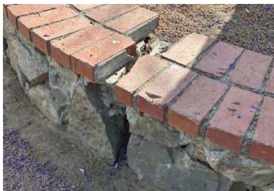
Detail at planter wall; note large separation and missing paver (ARG, 2023).
