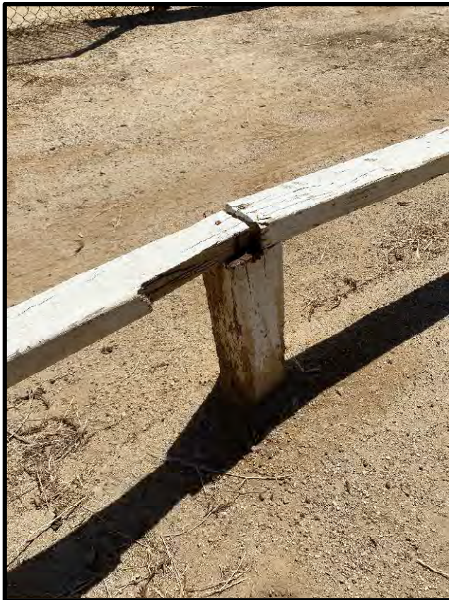
Figure 41 View of significant wood deterioration at the Internal Guide Rails.
