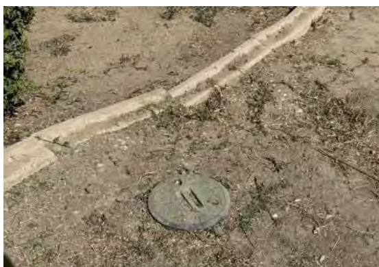
Detail of shifted curbs (ARG, 2023).
