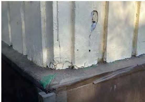
Detail at northeast corner; note wood decay and peeling paint at base of siding; also note loss at wood sill (ARG, 2023).
