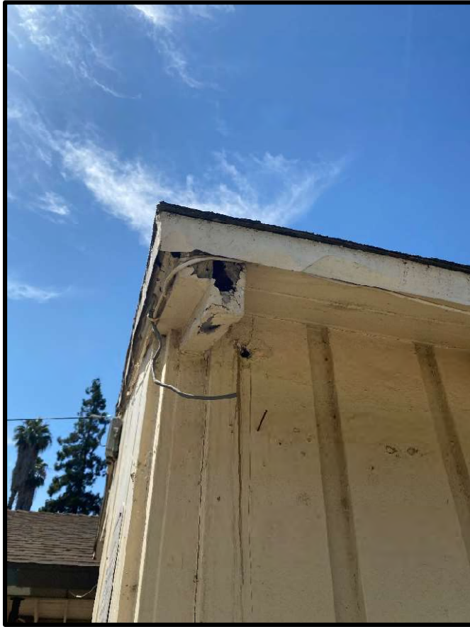
Figure 38 View of the roof rafter deterioration at the ends of the member.
