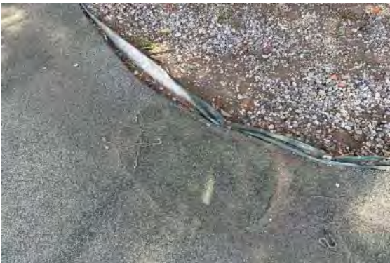
Detail at rubber floor ring; note soiling and low spots (ARG, 2023).
