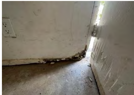
Detail at base of door interior; note door and wall damage (ARG, 2023).
