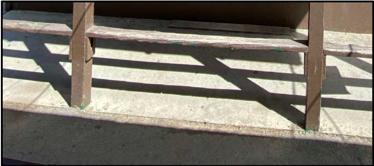
Figure 40 View of minor biological growth and insect damage at the base of the Ticket Booth columns.
