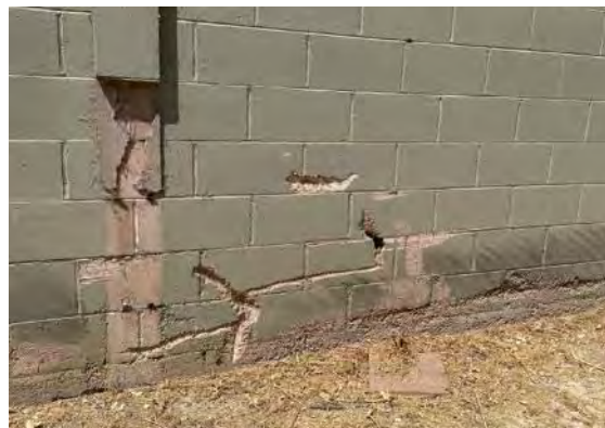
Gouges at base of CMU wall (ARG, 2023).
