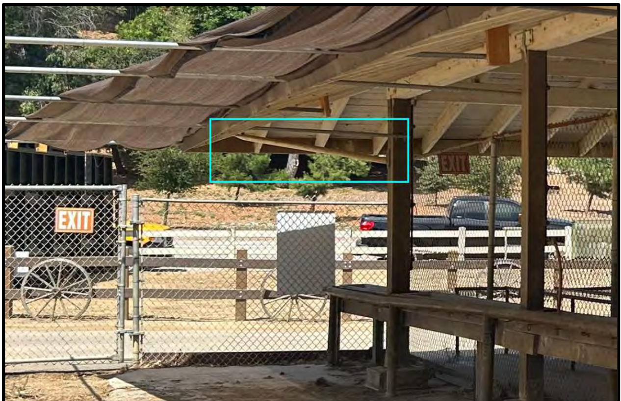
Figure 2 Steel tubes that appear to have been added to the Pergola.
