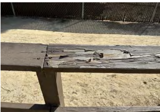
Typical peeling paint at buggy track fence (ARG, 2023).
