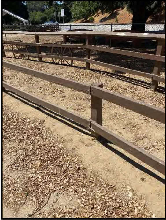
Figure 27 View of the Running Guide Rail.
