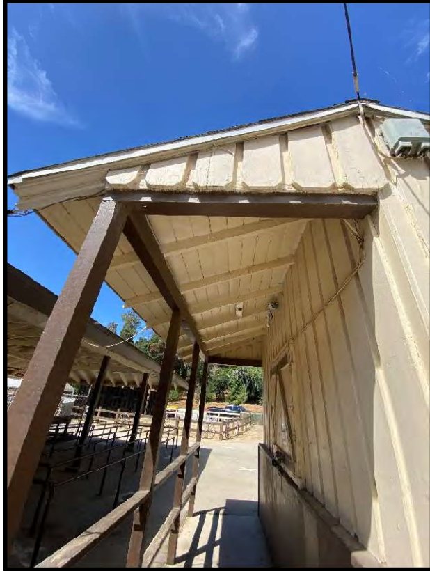
Figure 23 View of the Ticket Booth roof framing at the south roof overhang.
