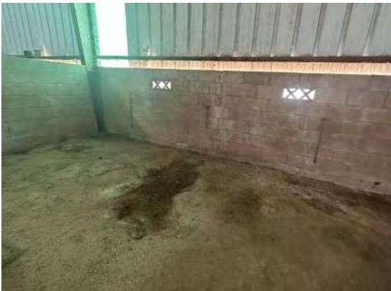
Detail at open area at south end; note staining and efflorescence (ARG, 2023).
