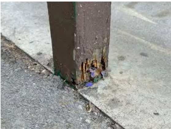
Detail at base of porch column; note wood decay/rot (ARG, 2023).
