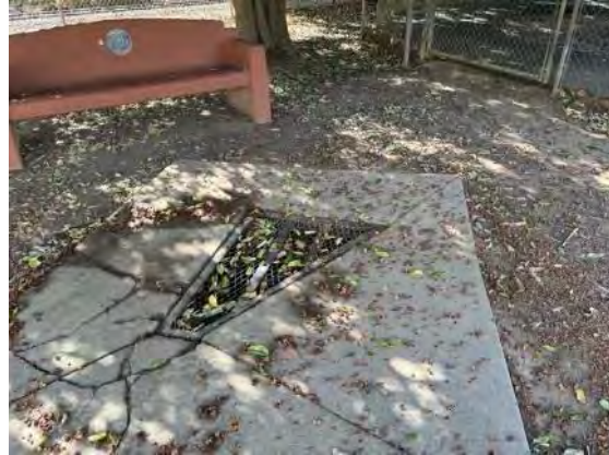
Concrete drainage structure near pony sweep; note cracking and debris (ARG, 2023).
